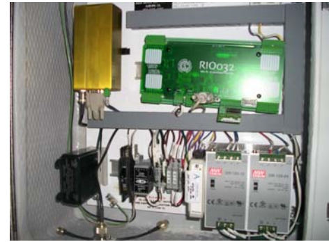
Telemetry equipment, which receives a reading of the tank level via radio frequency and controls the well pump
